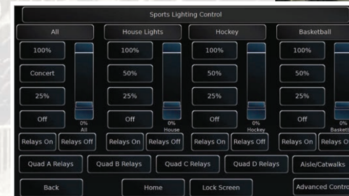
Sports Lighting Control
